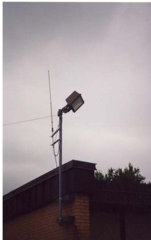
The antennas on Burbank School
